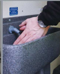
Delivery of hot water
